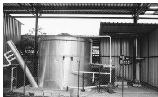
BIOGAS PLANT AT RESTAURANT
